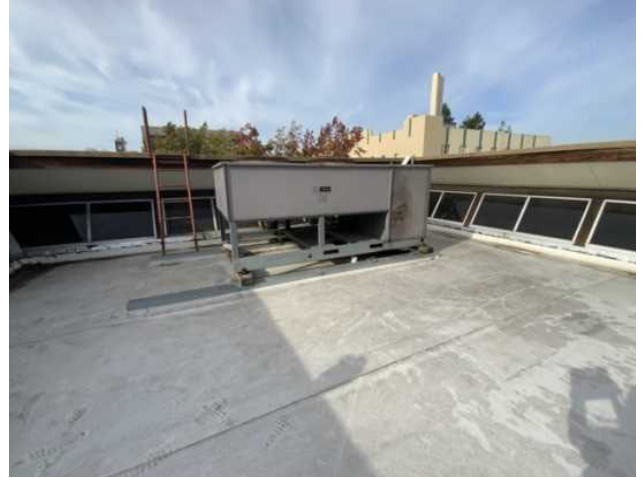
20 - ROOFTOP SPLIT SYSTEM UNIT
