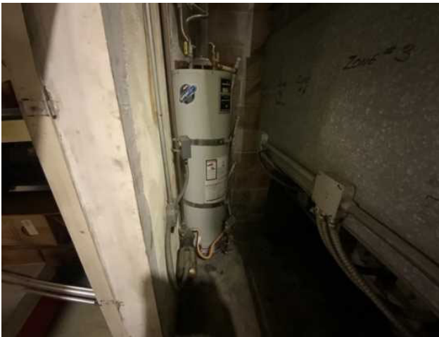
15 - GAS WATER HEATER
